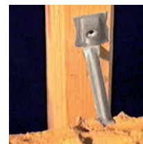
In light frame construction this can become a real problem especially on lower courses with semi cured mortar
